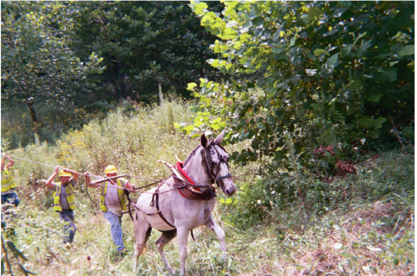
Employees of Foothills Rural Telephone Cooperative use a horse to lay fiber in rural Johnson County, Ky.
